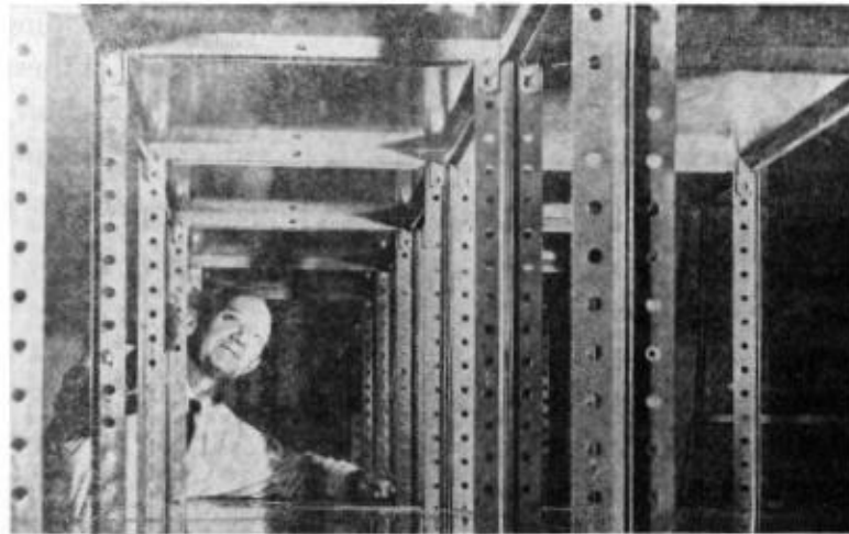
Joseph N. Nemelka, center supervisor, inspects steel shelving to hold additional Church records, Church Historian's Office.
